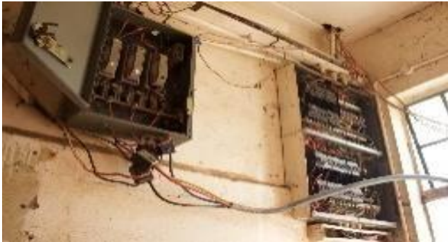
Just some of the dangerous wiring that is threatening the hospital
