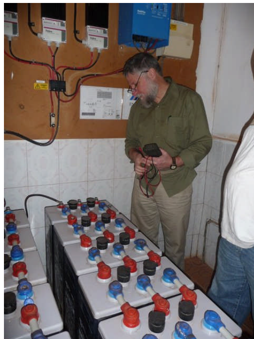
Leland from PUG checking batteries
